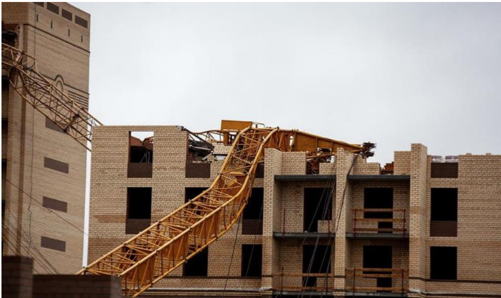
Fig. 1–Tower crane stability loss
