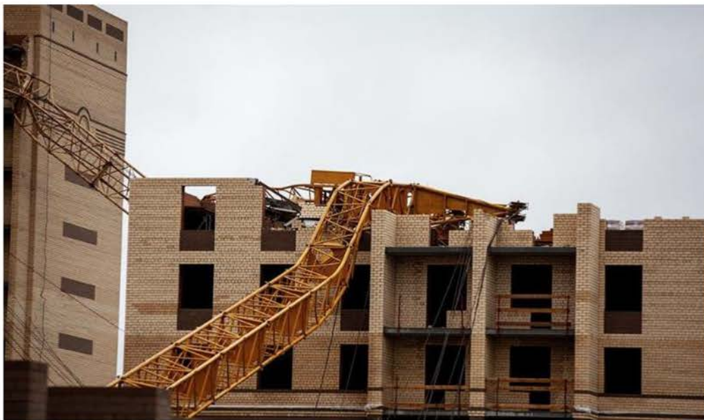
Fig. 1–Tower crane stability loss
